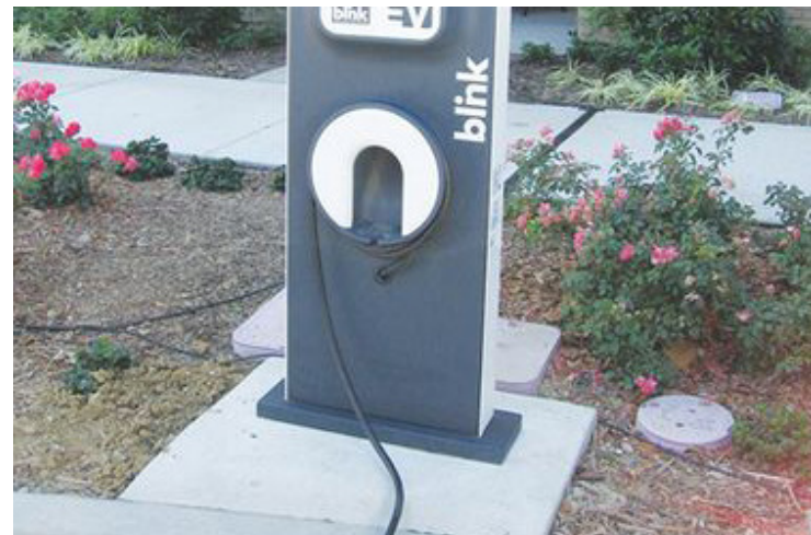
Standard 3.6.d: Charging station shall be a minimum of 24 inches clear from the face of curb.
