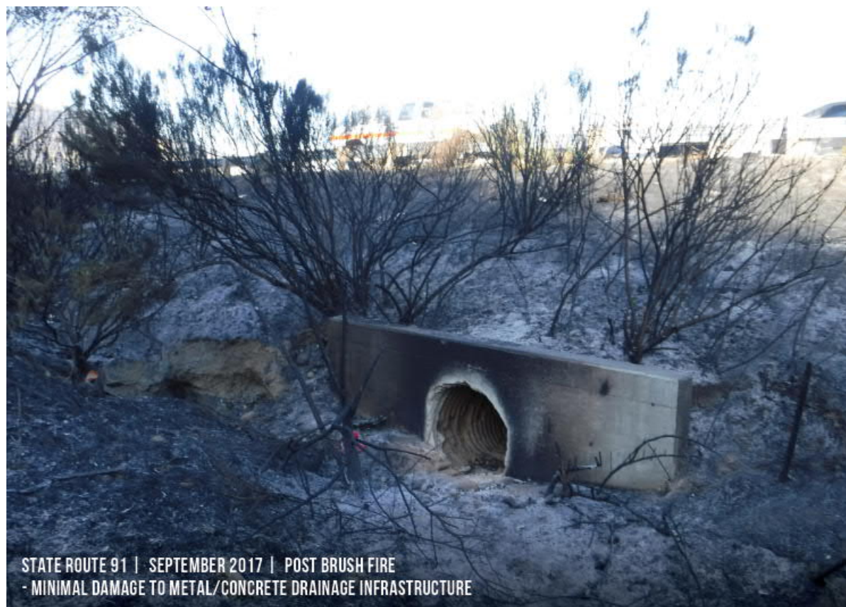
Figure 5 - Metal Pipe and Concrete Headwall Post-Fire
